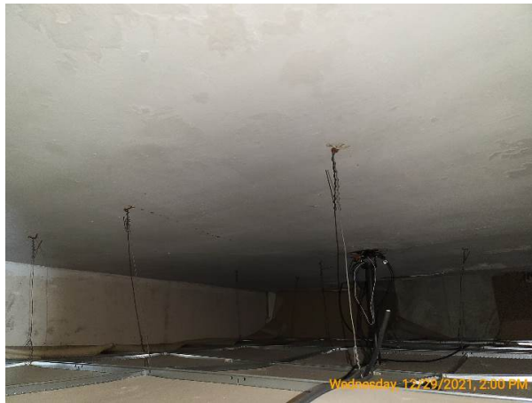
Plaster ceilings above the kitchen drop down
