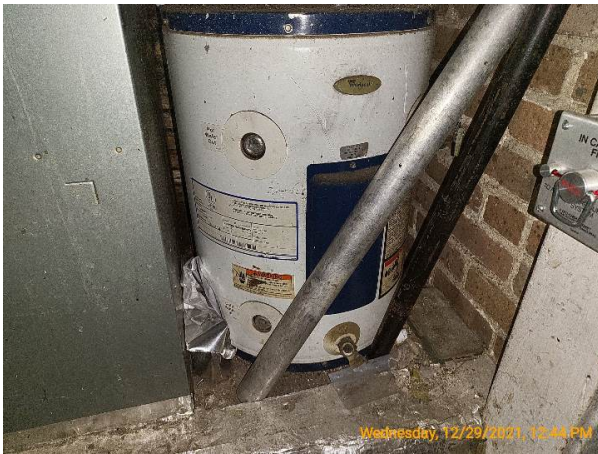
12 gallon electric water heater manufactured in 2008, functional
