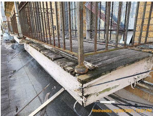
All balcony roofs are in poor condition
