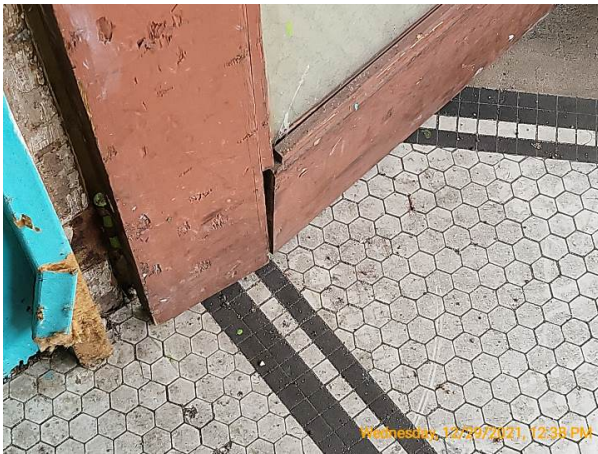
Same door significantly damaged at the bottom
