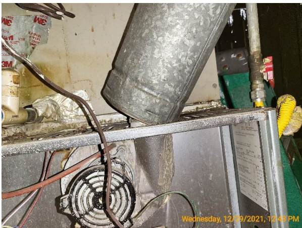
Unsafe to use because vent is disconnected and improper
