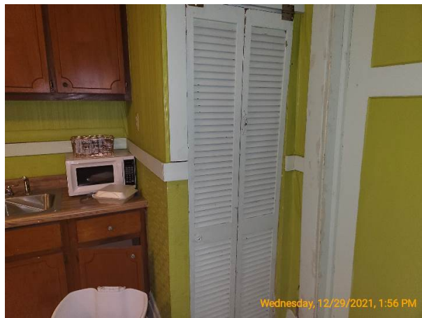
Gas water heater is not accessible
