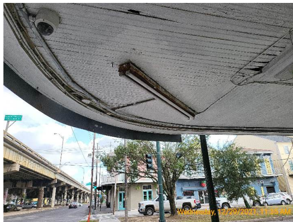
Overhang lighting was not functional
