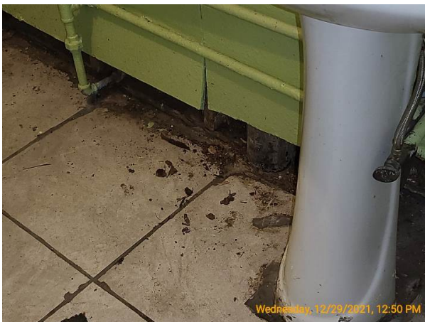
Severe framing damages at the base of the wall in the men's restroom
