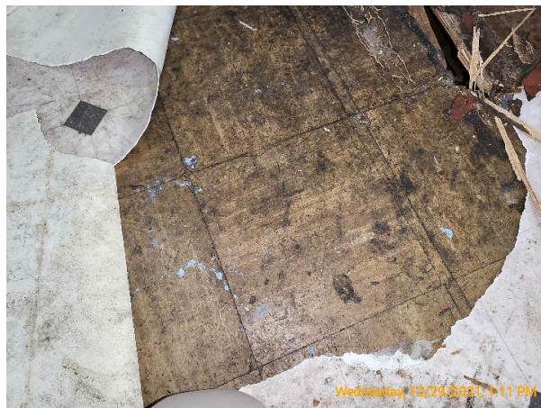
Possible asbestos tiles under the vinyl floor
