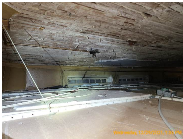
Crown molding intact along the left wall below the beams, which suggests they are still functional
