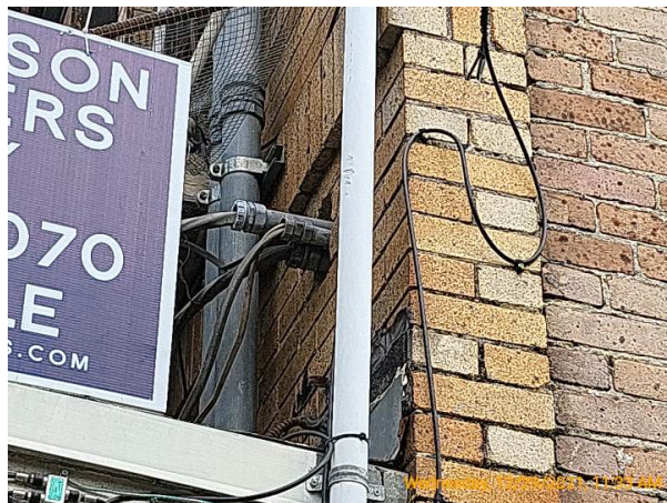
Electrical wires are not in conduit at the right front corner
