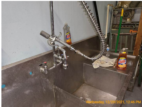
Water flow reversed
