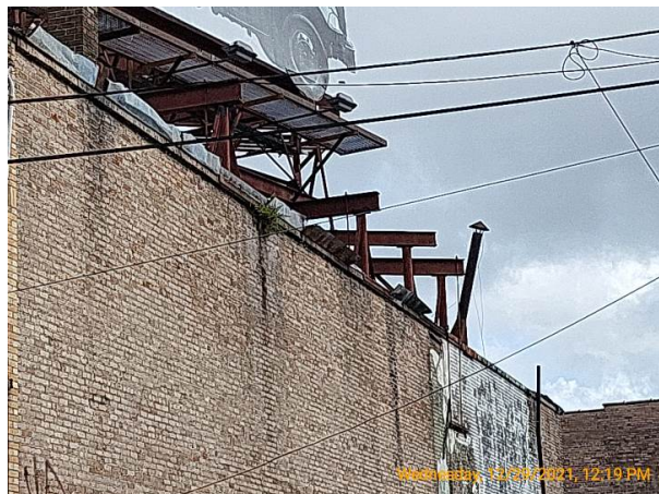
Severe vegetation growth along the right side
