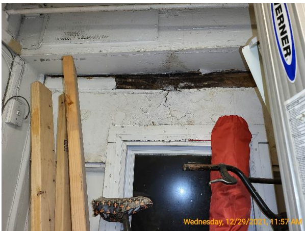
Severe moisture damages and rotted wood at the filled in cased opening at the equipment closet
