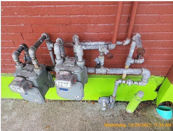
Four gas meters enter at the left side, two have been removed and two are on
