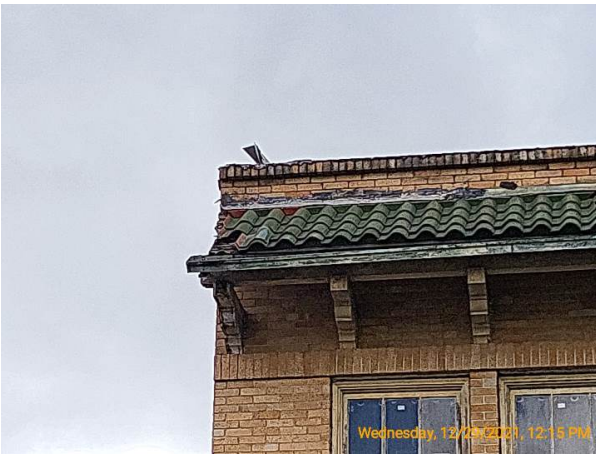
Terracotta tile roof failing around the left and front of the building
