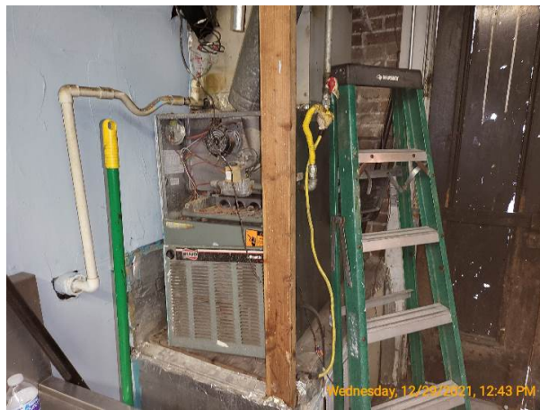
Inoperable gas furnace and coil over 10 years old
