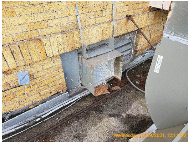
Old vent opening should be removed
