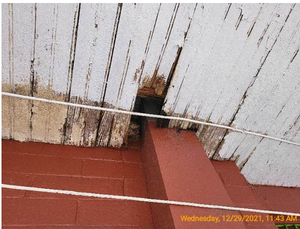
Significant wood rot below the sidewalk overhang
