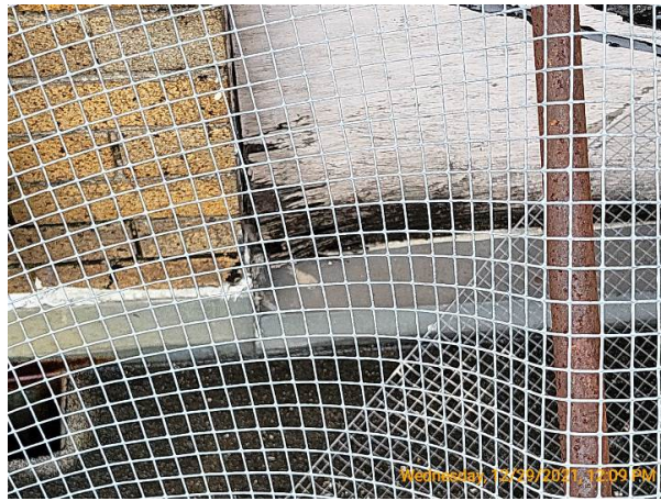
Rotted wood panels at masonry openings
