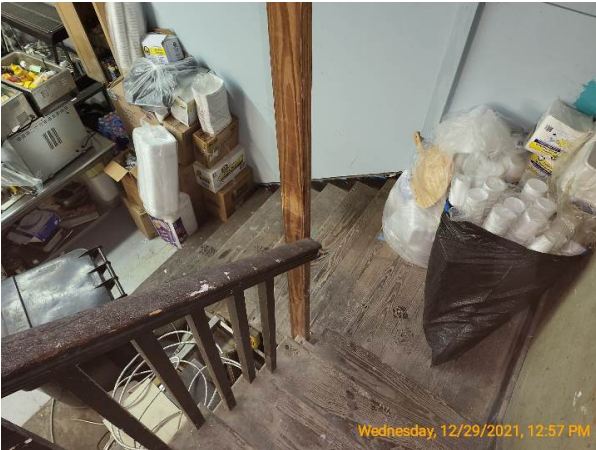
Loose railing and missing railing at the stairs to the second floor
