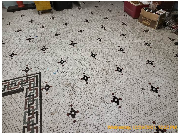
Typical cracking in the floating slab
