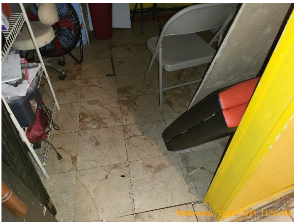
Raised wood floor rotted
