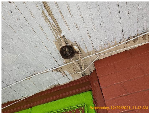
Cloth Romex and open junction box
