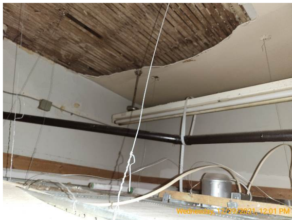
Drop down ceiling marginally supported, plaster prevents view of beams
