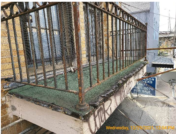
Representative failing roof at all balconies
