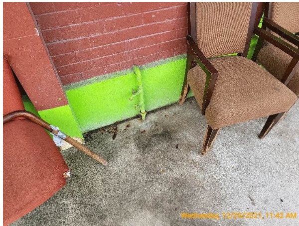
Single water meter enters at the left side
