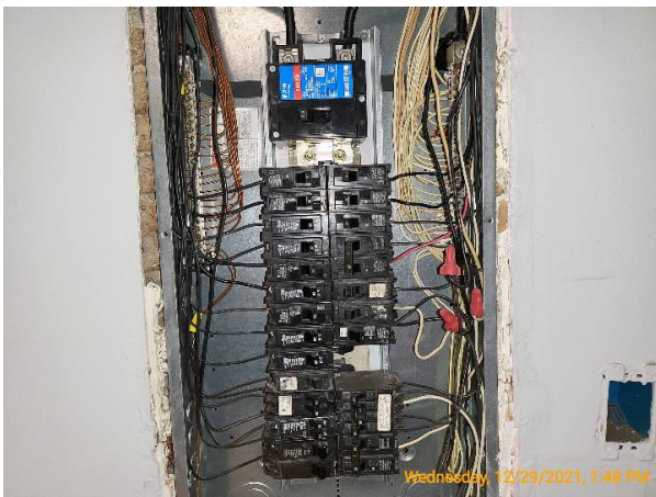
Main electrical panel
