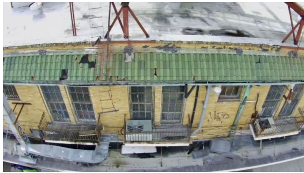
Terra cotta tile roof missing numerous tiles
