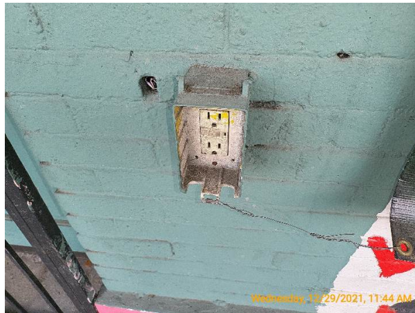
Another missing weather cover
