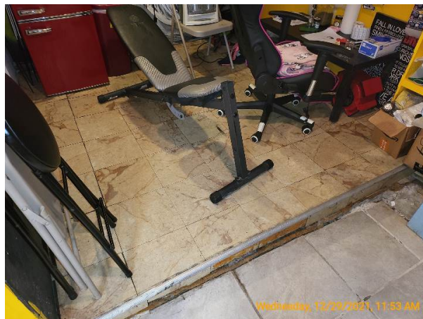
Another raised wood floor rotted through
