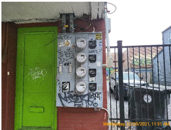
Four electric meters at the right front corner with service disconnects
