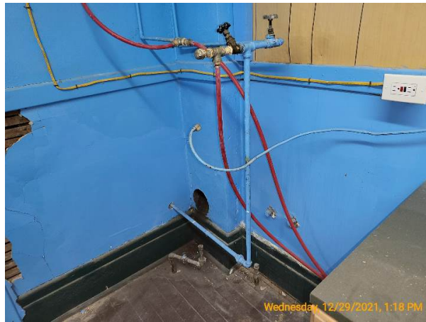
Water heater not installed
