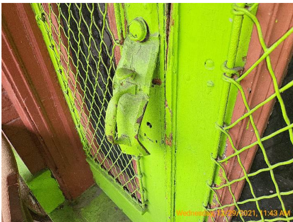
Damaged door lock at the left side marked 1630
