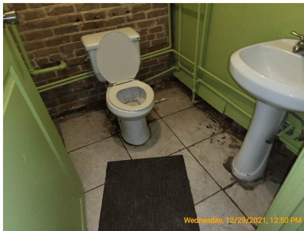
Loose toilet in the men's restroom
