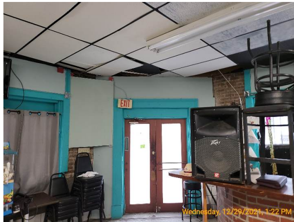
Inoperable emergency exit lighting for unit 714
