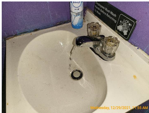
Severely low water flow in the half bathroom
