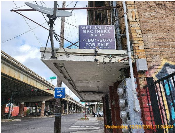
Sidewalk overhang has a negative slope across the front
