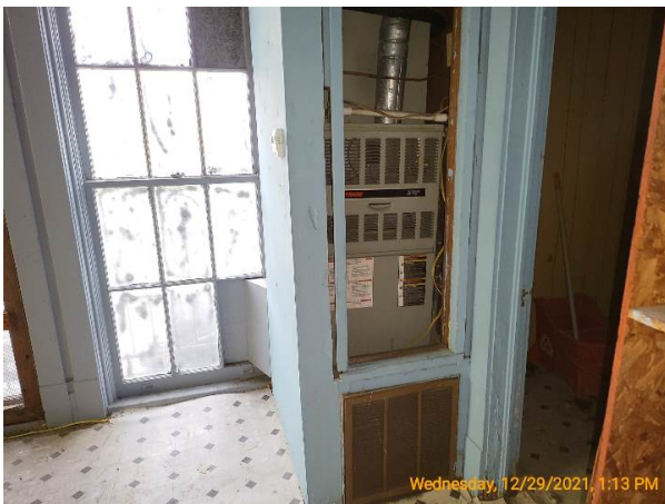
Inoperable furnace and heater that appears to be over 15 years old
