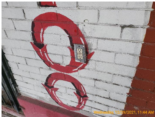
Missing outlet cover
