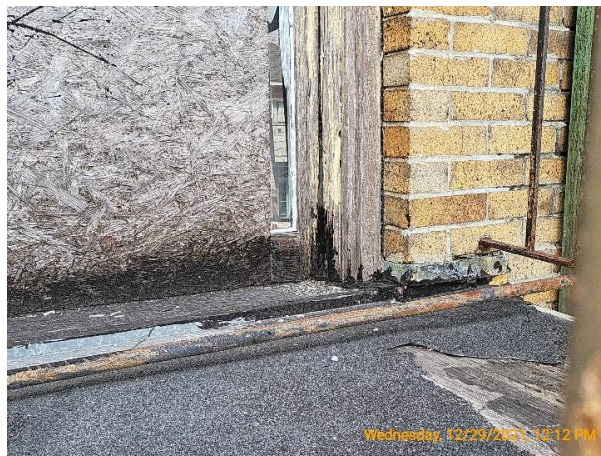
Rotted window sashes and sills noted
