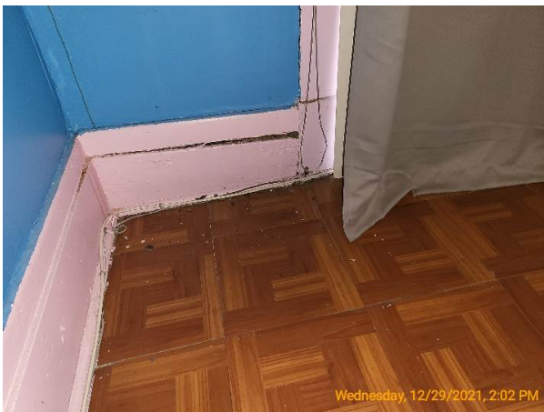
Significant deflection and split baseboard over the tattoo place, indicative of hidden beam damage
