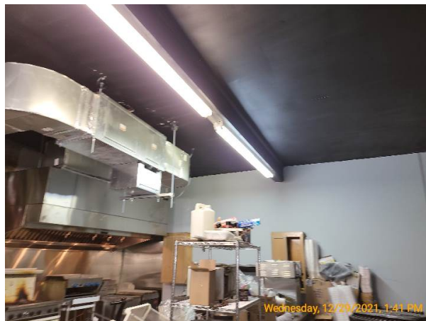
Plaster ceiling intact at the rear half of 714 and no visible beams
