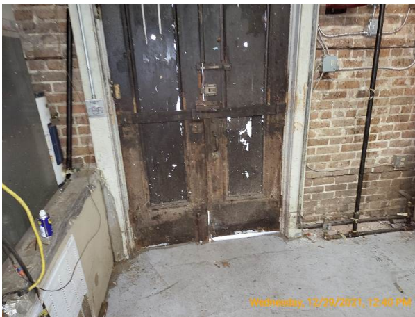
Another damaged door
