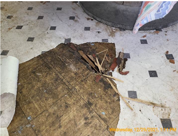
Significant subfloor and visible framing damages at the left front corner of the building
