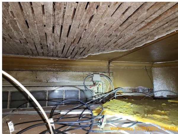
Open junction box
