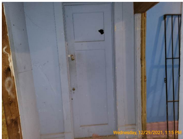
Inaccessible closet opposite the bathroom after front
