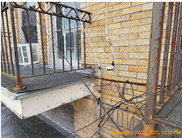
Exposed and loose electrical wiring
