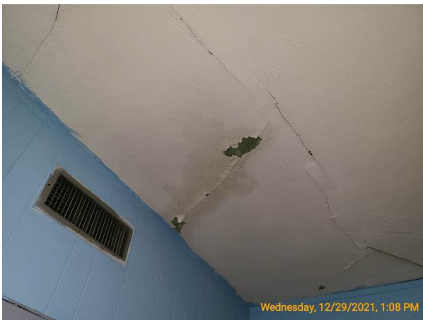
Significant moisture staining on the second floor ceiling
