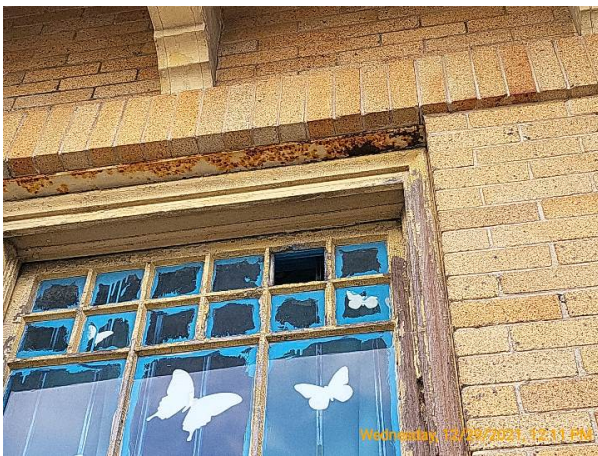
Missing window pane
