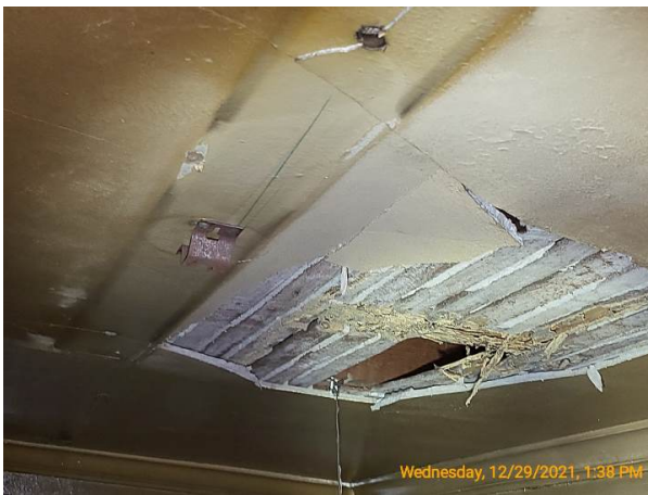
Significant damages at a right side beam 714
