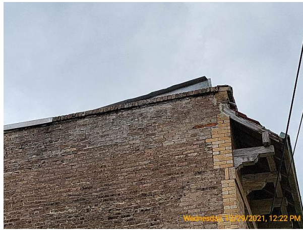
Parapet cap missing along most of the building
