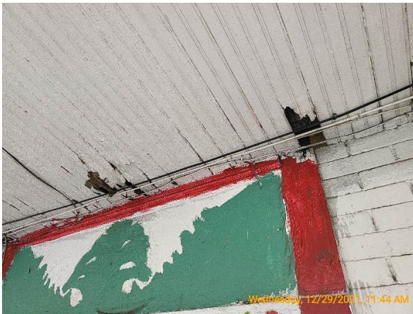
More soffit rot at the left side sidewalk overhang
