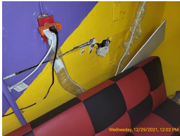
Severe moisture damage is below the window unit
