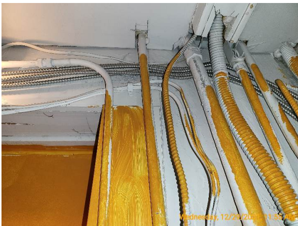
Exposed electrical wire
