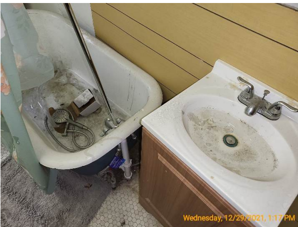
Slow drain at the rear bathroom sink and tub
