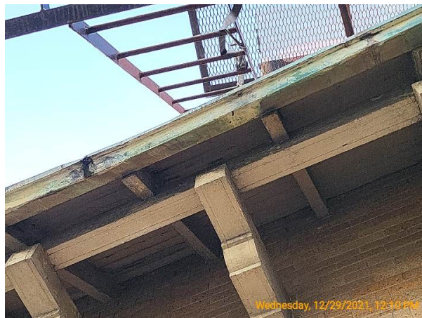
Upper copper gutter is failing
