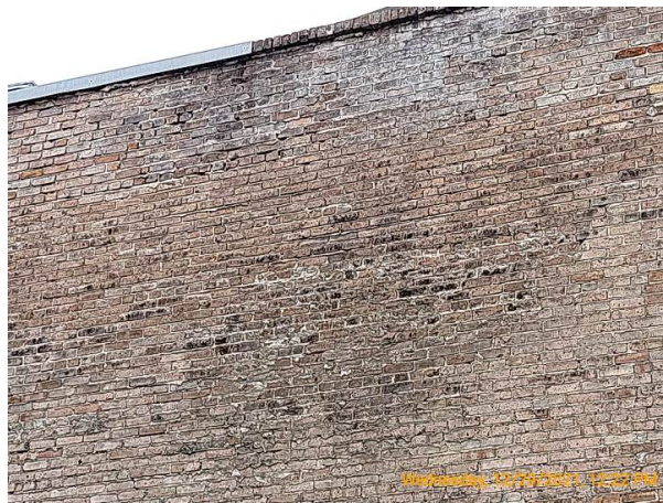
Numerous holes were noted in the mortar in the rear wall
