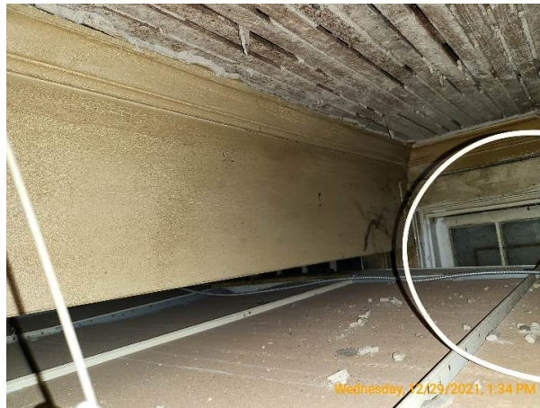
Central beam 714 appears functional
