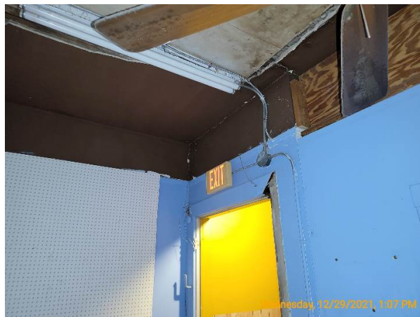
Emergency exit lighting is present but no corridor lighting is present
