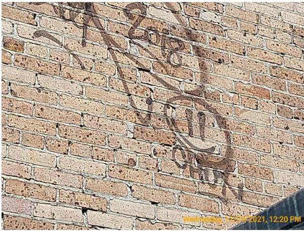
Numerous holes in the mortar were noted along the right side
