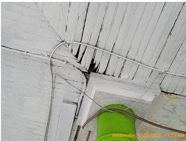
Significant wood rot below the sidewalk overhang
