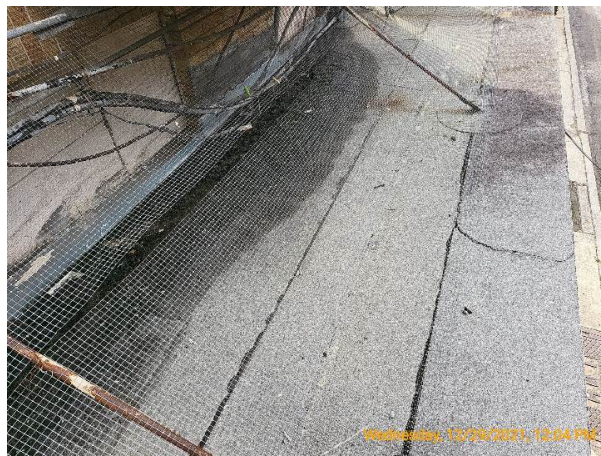
Severe water pooling at the building side of the sidewalk overhang
