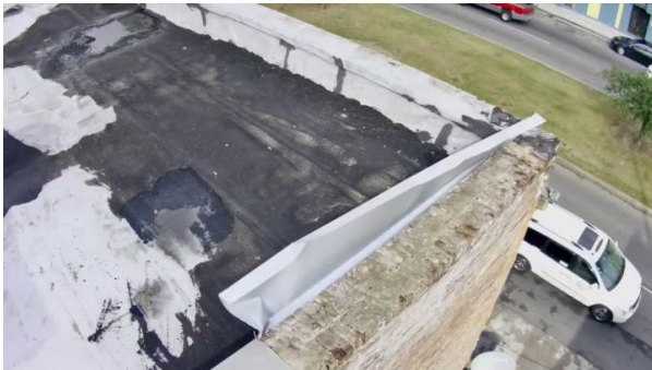
Damaged parapet cap
