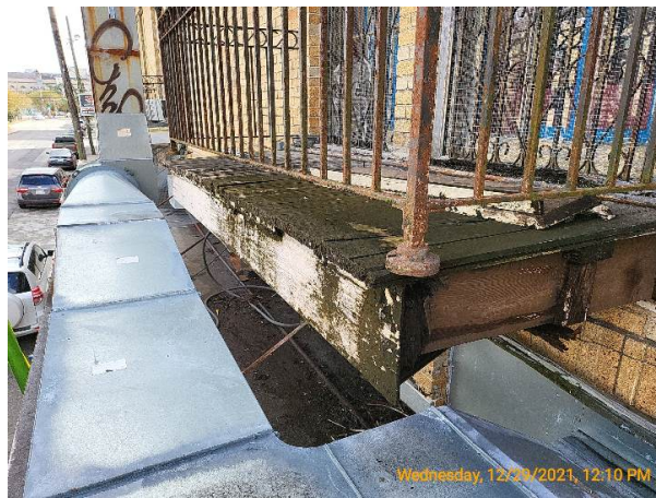
A left side balcony is notably out of square and structurally failing
