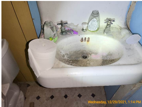
Inoperable hot water fixture
