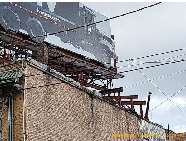
Metal parapet cap along the right side are bent upwards and significantly damaged
