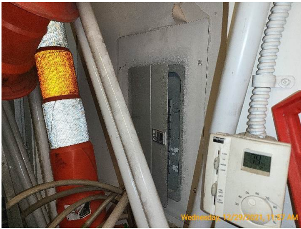
Sub electrical panel not accessible
