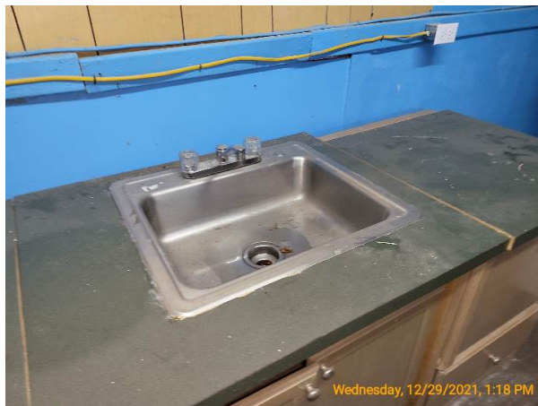
Kitchen sink has a slow drain
