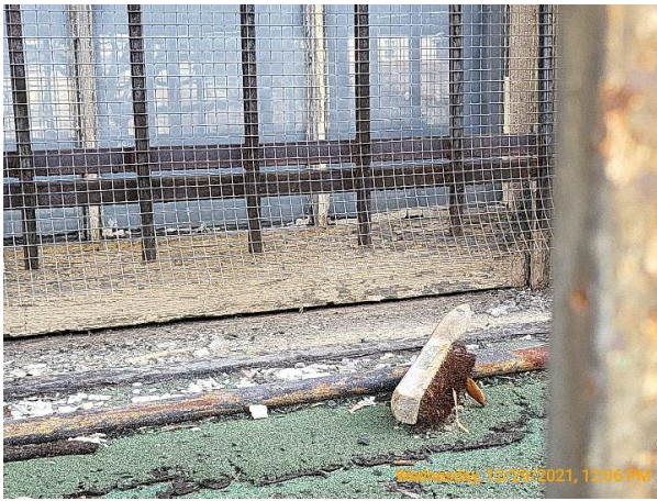
Significant glazing cracking and paint flaking at the windows
