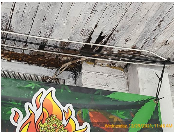
More exposed electrical wire, Significant wood rot below the sidewalk overhang
