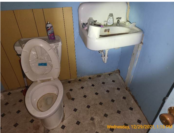
No water heater
