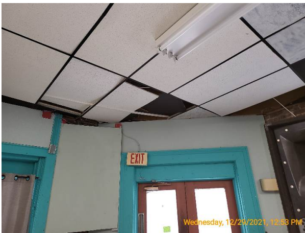
Significant ceiling tile damages throughout the entire first floor
