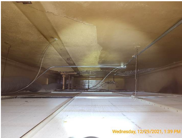
Plaster covers most of the right half ceiling of 714
