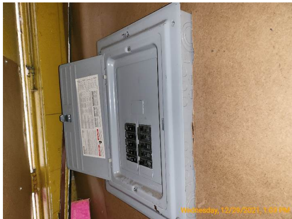
Sub panel for unit 712
