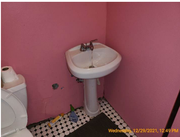
Loose sink in the women's restroom
