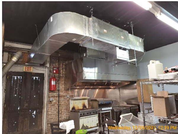
Fire suppression and vent system added, it was a $40,000 upgrade
