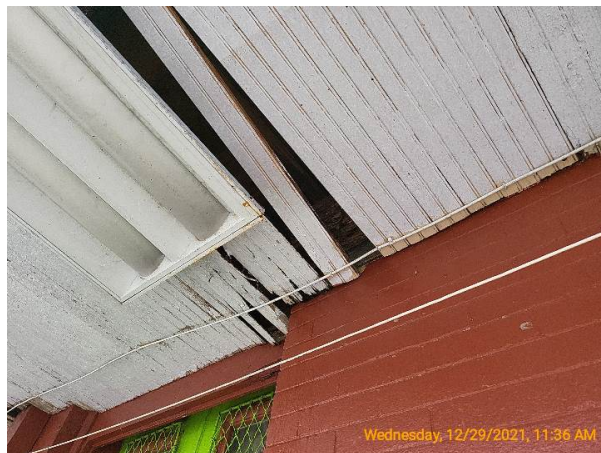
Significant wood rot below the sidewalk overhang
