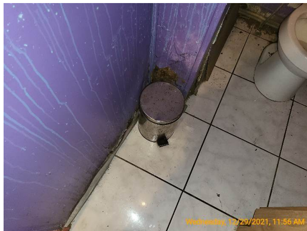
Severe moisture damage and possible mold growth at the base of the half bathroom wall
