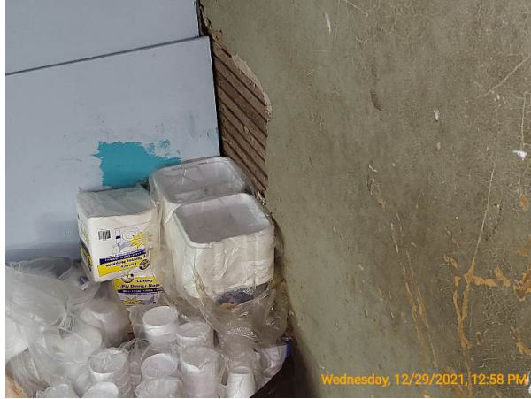
Missing plaster throughout the exterior walls
