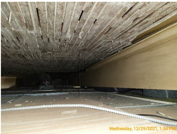
Central beam 714 appears functional
