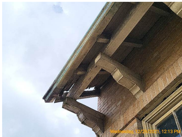
Upper roof soffit rot
