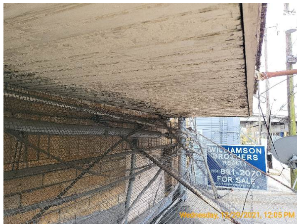
Severe wood rot and moisture staining below a front balcony
