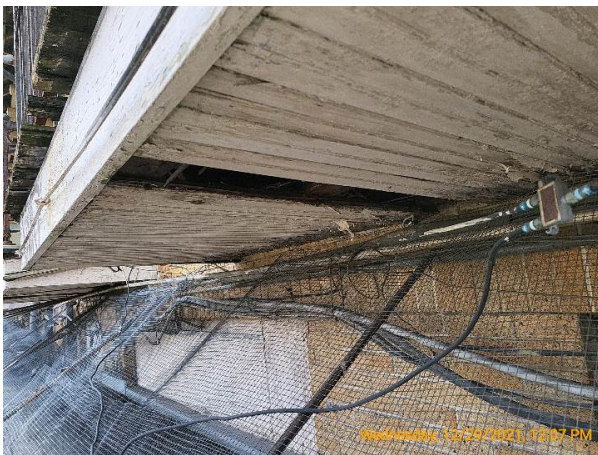
All balcony roofs have severe wood rot and moisture staining below them
