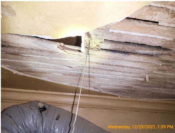
Significant damages at a third beam over the right half of 714
