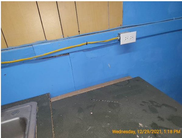
Newer electrical wiring not in conduit
