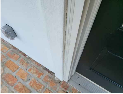
Door sealant separation
