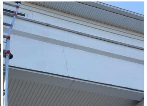
Notable crack over the front stairs and we recommend removal of the trim to evaluate the beam
