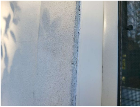
Separations noted at the window sealant
