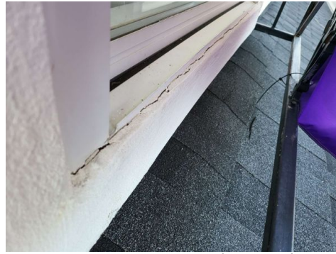
More separations at another window
