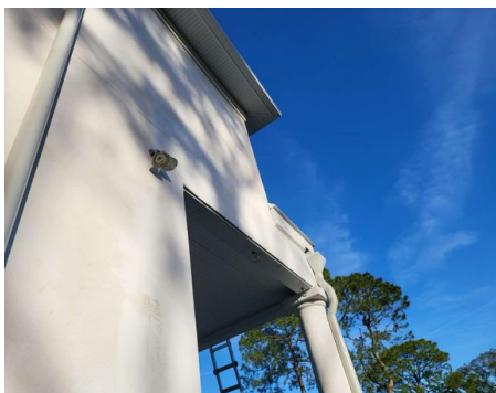
Based on the color difference in the stucco it appears that repairs were done to the front porch beams
