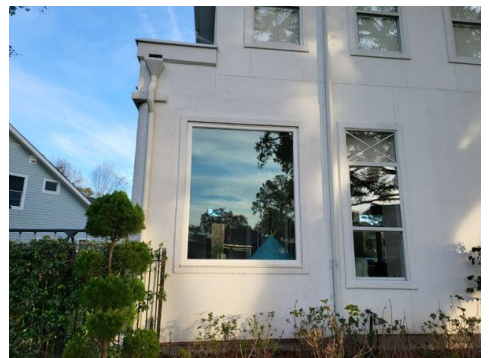
Grind crack and seal at the right rear corner of the house at what looks like an enclosed porch
