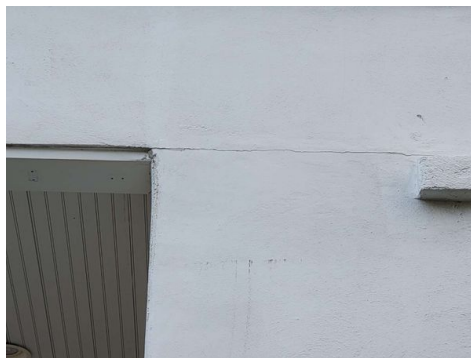
Close-up showing the location of the crack
