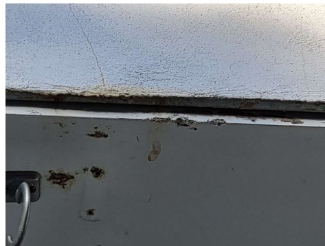
Chronic calcification at the base of the stucco and moisture staining on the wood trim below the left side beam, we recommend removal of the trim to evaluate the beam
