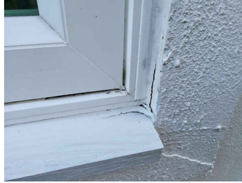
More window sealant separation
