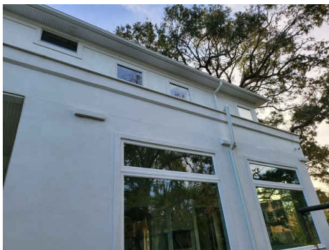
Grind crack and seal between first floor wall and second floor roof wall junction
