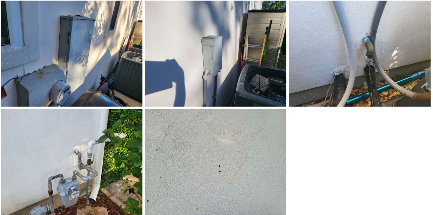
Seal various holes in the stucco near the windows that we suspect are old shutters
