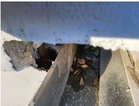
Large hole in the stucco at the left front corner should be waterproof
